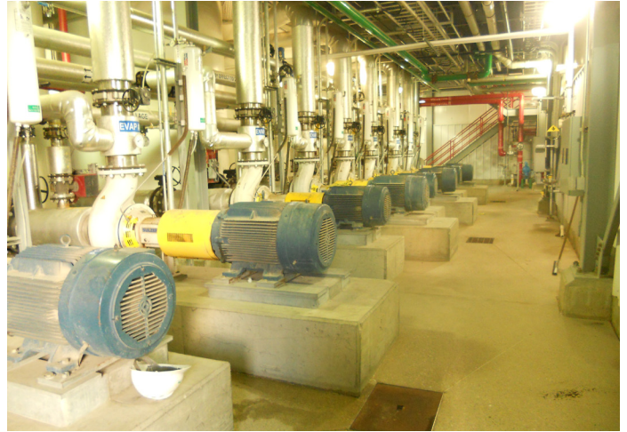
The plant saves around $28,000 per year through sales tax exemptions on energy that powers equipment used directly in ethanol production, such as these high-efficiency evaporator and condensate pumps.
